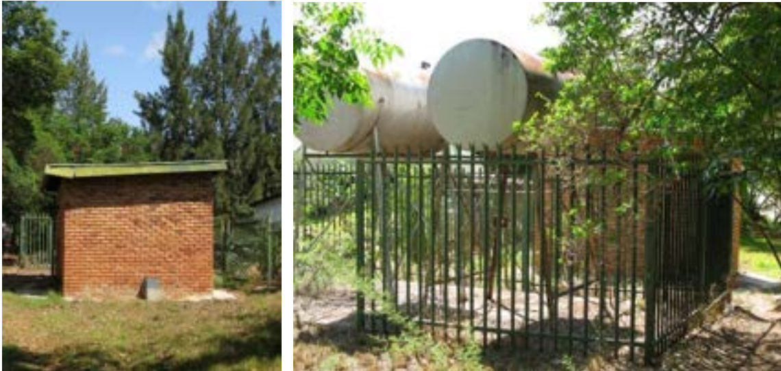
Figure 37: The generator storeroom (left) and the diesel storage tank for the generator (right)
