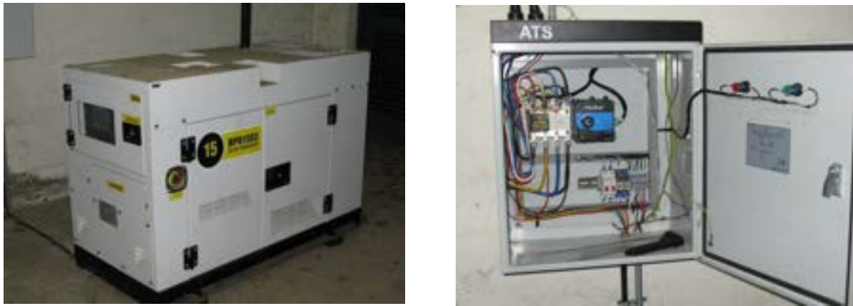
Figure 59: Back-up generator for the marine research facility (left) and the electrical panel with the automatic changeover switch (right)
