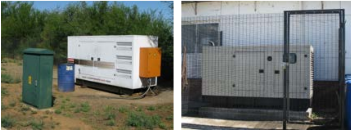
Figure 108: The generator for the administration block (left) and the generator for the farm (right)
