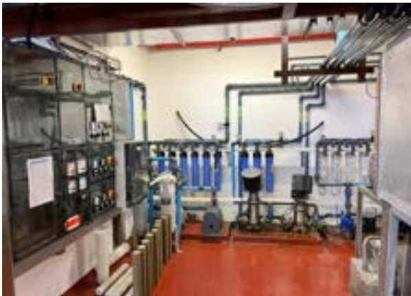
Figure 124: Filtration systems in place
