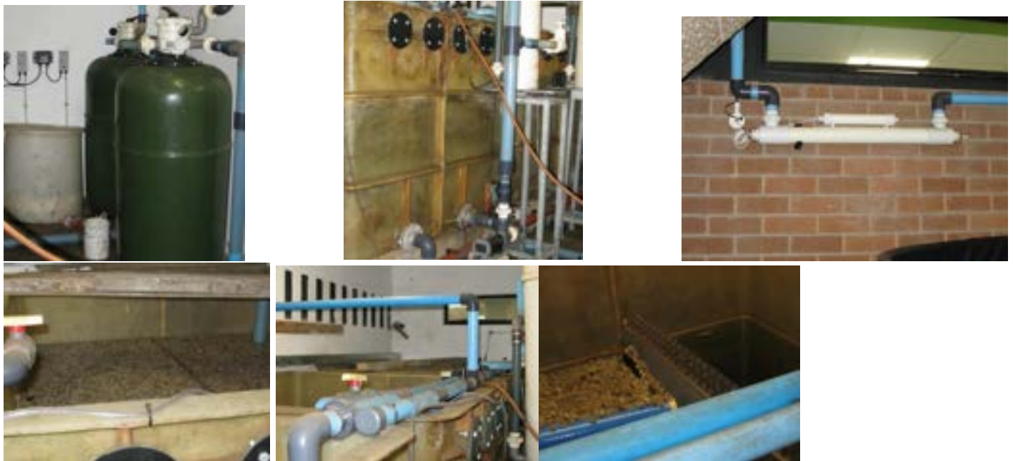
Figure 60: Filtration systems, including sand filtration (top left), tickle biological filter (top middle), UV sterilization unit (top right), biomedica in the biological filter (bottom right), and more biological filter and biomedica (bottom)
