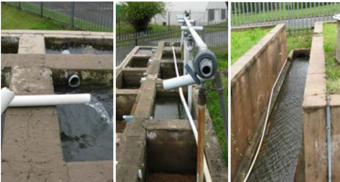
Figure 53: Biofilter inlet (left), main biofiltration channel (middle) and wastewater channel (right)
