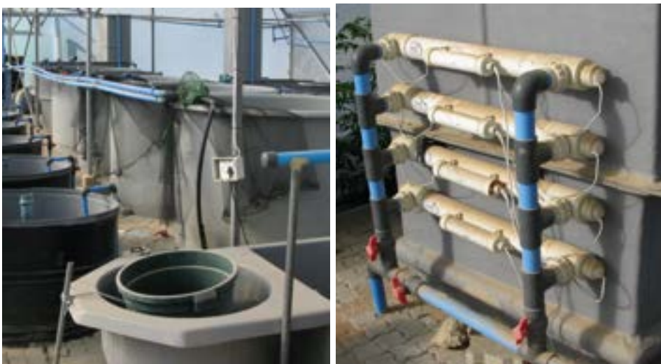
Figure 77: DARDLEA facility experimental tanks and UV sterilisation system
