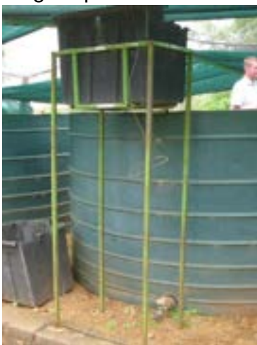
Figure 85: Simple water filtration system that is no longer functional
