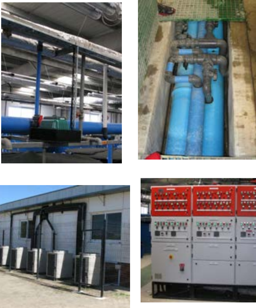
Figure 112: Water and air reticulation (top left), RAS pipework canal (top right), heat pumps (bottom left) and main electrical panel (bottom right)
