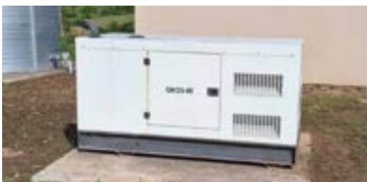
Figure 118: Back-up generator on site
