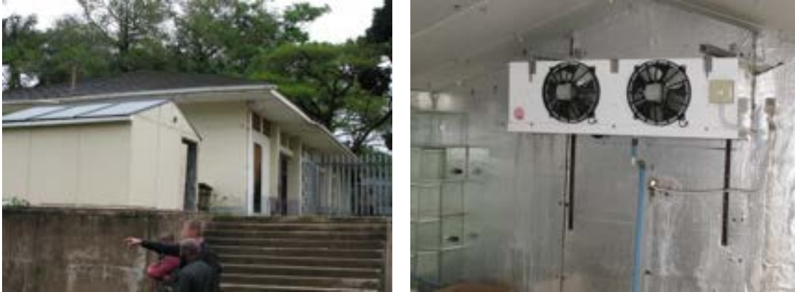
Figure 54: Feed storage facility (left) that is temperature controlled with chillers (right)
