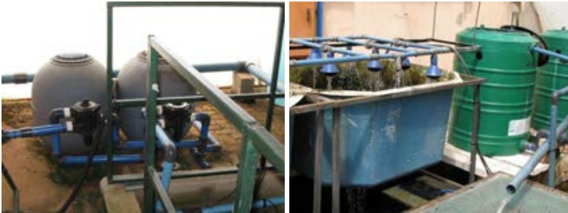
Figure 40: Filtration system for the ornamental facility with sand filters (left) and a trickle biological filter (right)
