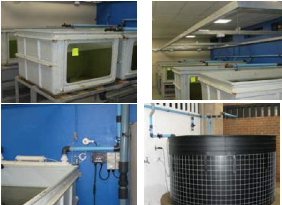
Figure 62: New systems installed as part of the marine research facility with fibreglass tanks (top row), pump controllers and monitoring sensors (bottom left) and round PVC-lined tanks (bottom right)
