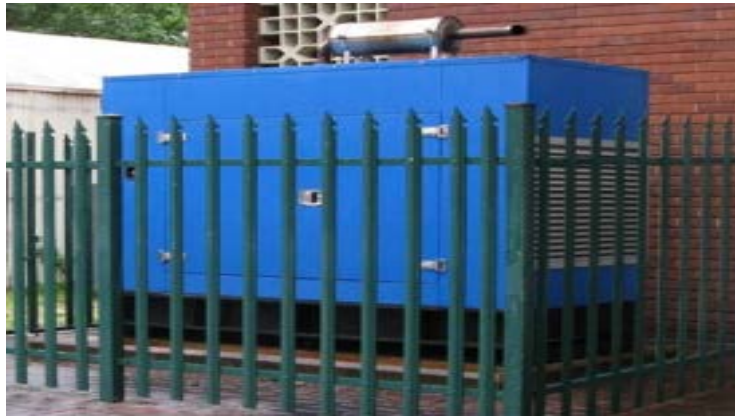
Figure 31: UKZN's Back-up generator
