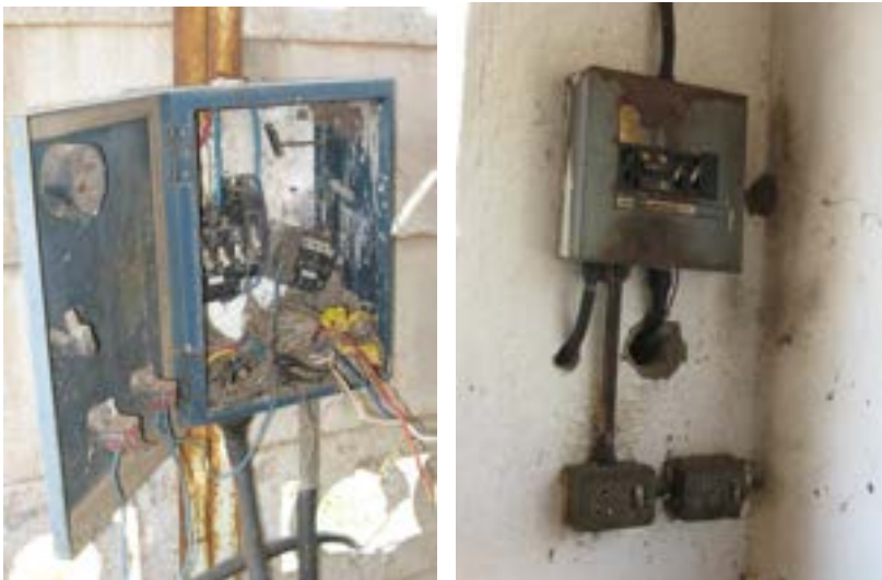
Figure 93: The state of the electrical boards at the aquaculture facility
