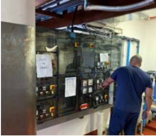
Figure 123: Main electrical panel
