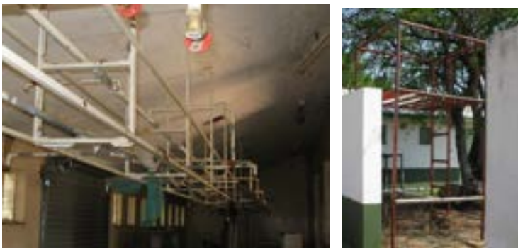
Figure 95: Non-functional life-support systems (left) and the scaffolding structure that once held a water reservoir (right)
