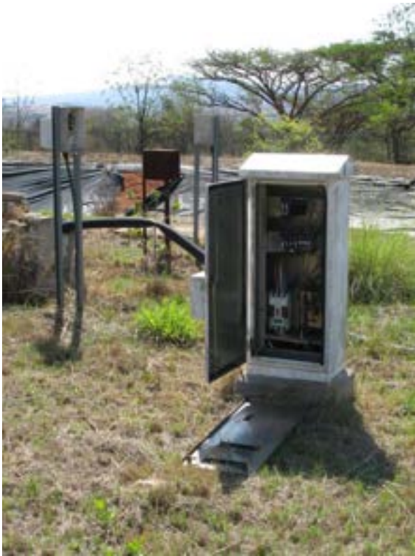
Figure 38: The electrical box for the new tunnel system
