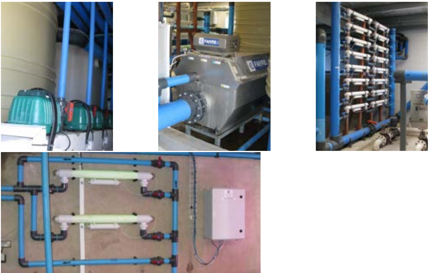
Figure 109: Filtration systems and pumps (top left), the drum filter (top middle), UV sterilisation banks (top right and bottom)
